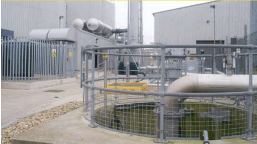
Budds Farm Sewage Treatment Works in Langstone Harbour
